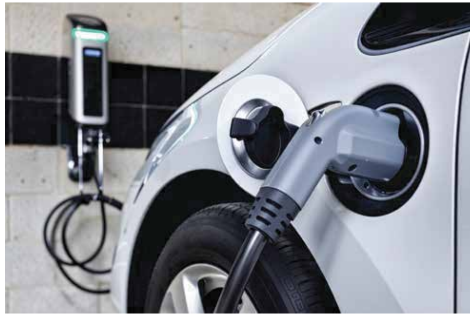
EV CHARGING FACILITY
